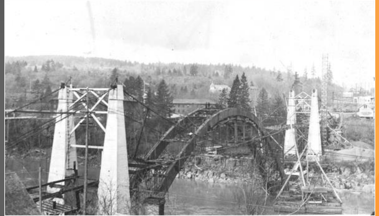
Towers of old suspension bridge used in construction of the Willamette River (Oregon City) Bridge in 1921-22.
